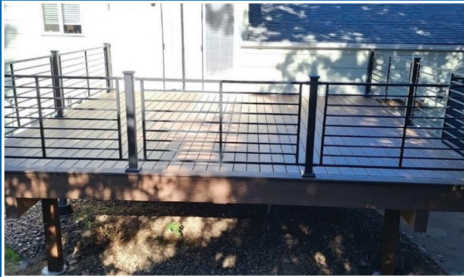
Figure 1: Completed wood build using Kiln Dried PT, Fortress Axis Railing and MoistureShield Vision Decking.
