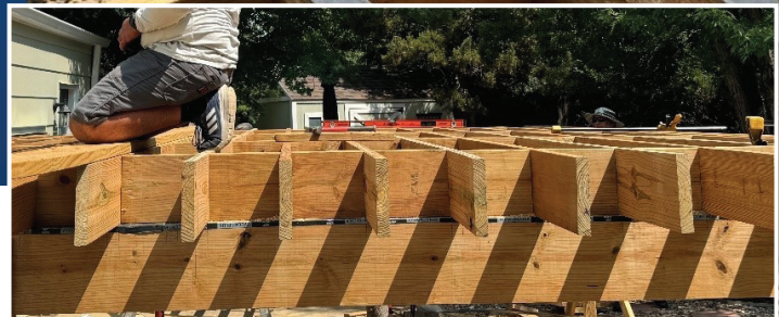
Figure 12: Builder installing the joist tape. Using a board to protect their knees and to make installing the tape easier.
